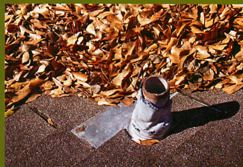
Squirrel Damaged Lead Jack Plumbing Vent.
