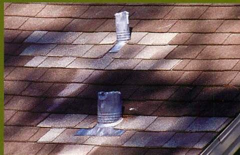
Typical repair for Squirrel Damaged Vents.
