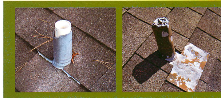
SquirrelGard™ may not provide a waterproof flashing repair.
